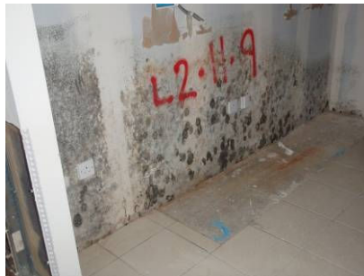
Toxic mould on plaster board
