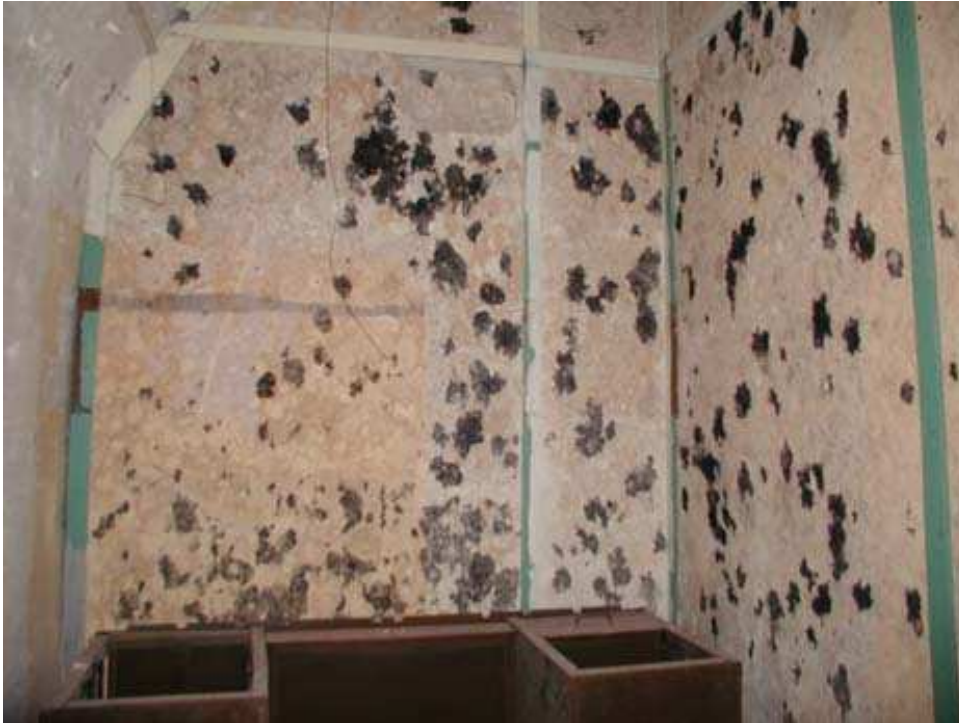
Mould growth on wall
