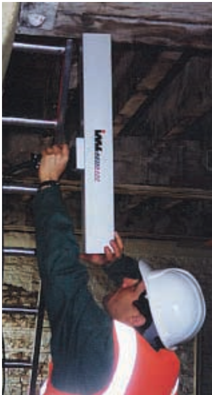
Figure 2 Use of the resistograph drill to inspect timber members (Environmental Building Solutions Ltd)
