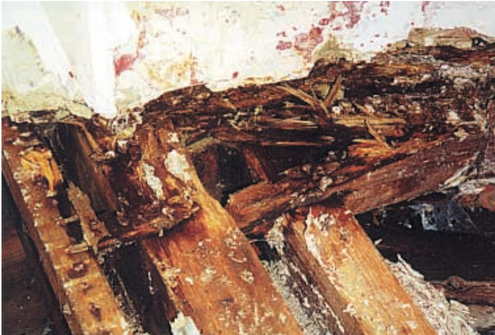
Figure 1 Timbers showing characteristic cracking and fungal growths associated with fungal decay (Environmental Building Solutions Ltd)
